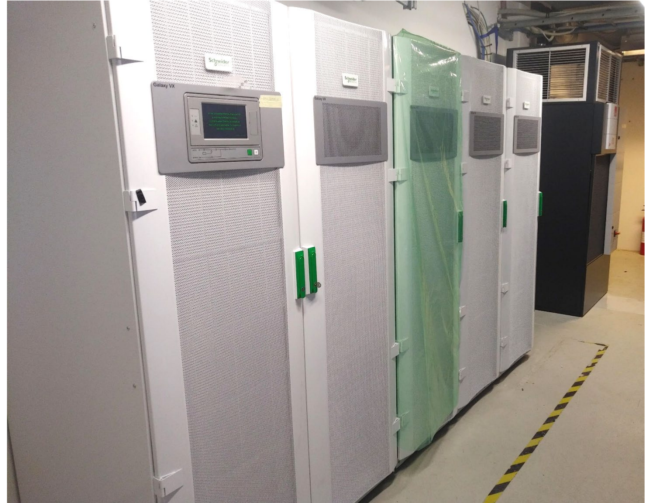
New UPS controller units + cooling unit
